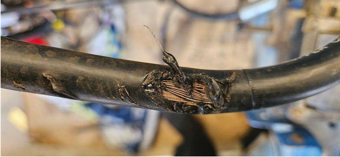
Figure 32: An image of a melted wire sheathing.
