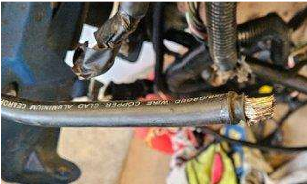
Figure 31: An image of a torn connection.
